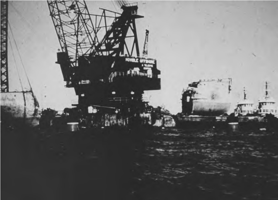
A 600-ton whirley crane lifts the stern section of the Corps of Engineers' dredge Mackenzie onto a waiting barge. The dredge's stacks still protrude from the water.
