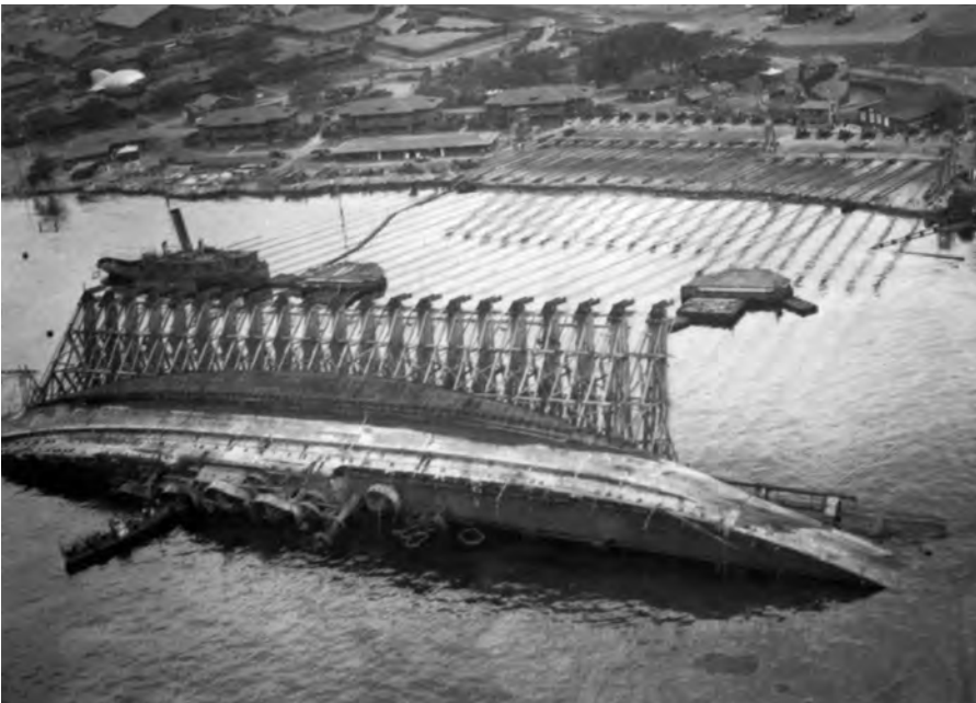
The capsized battleship Oklahoma was righted by building headframes on her side and pulling with purchases and winches mounted ashore on Ford Island.
